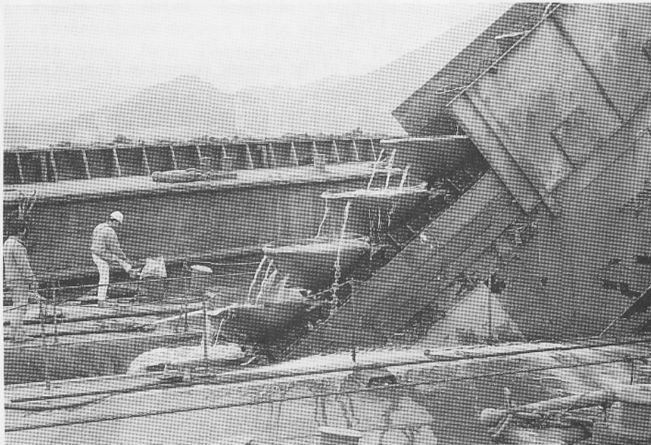
Dredging the trench for the Eastern Harbour Crossing in 1987. Source of the shell sample analyzed by Yim et al (1990). Photograph courtesy of R Shaw
